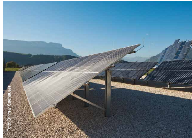
Overview of the multi-technology experimental PV test installation.
